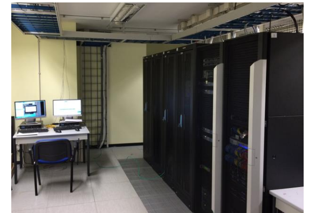
Server Room (BB-HUB, Servers, Network)
